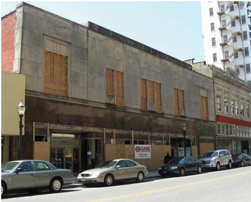
Hargrove and Associates is renovating the old Neisner's building on Royal Street and a portion of the Kress building for offices to house its 200 engineers and support employees. They will move in by the end of the year.
